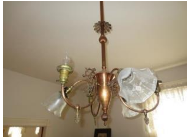
Light fixture wired for electricity and gas
